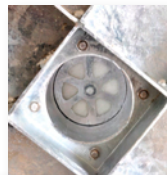
Filter insert inside the chimney
