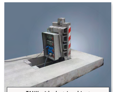
TANK with electric cabinet
